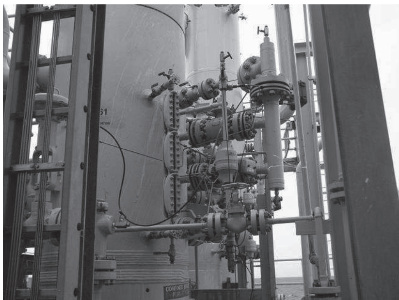
Figure 4: Example of Scrubber Attachments
