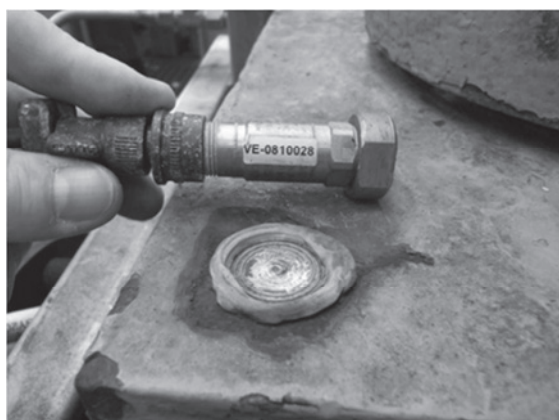
Figure 1: Broken vibration sensor – mounting base detaches from glue
